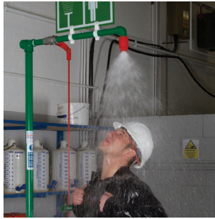
Emergency Safety Showers
