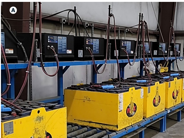
Violation: no emergency equipment available where chemicals are present or in use.
