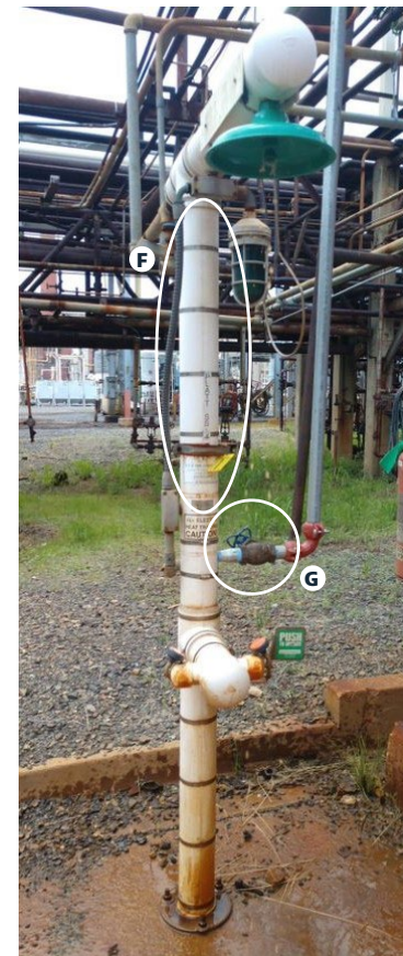
Violation: insulation added, not designed for outdoor use, no lock out/tag out on valve.
