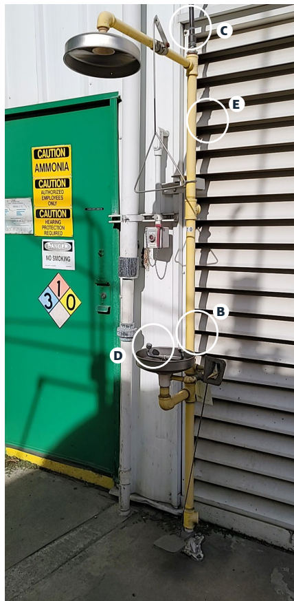
Violation: no scald protection valve, supply line is too small, no dust covers on eyewash, no signage.
