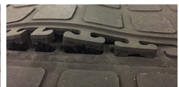
B) Waving mats are a trip hazard
