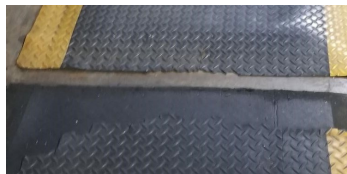
A) Worn tread is ineffective
