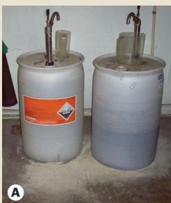
Violation: Hazardous liquids, no spill protection
