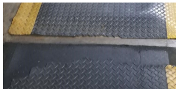
A) Worn tread is ineffective
