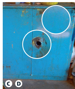
Violations: Missing handle and required label
