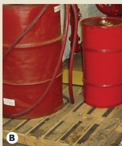
Violation: Not compliant spill pallet
